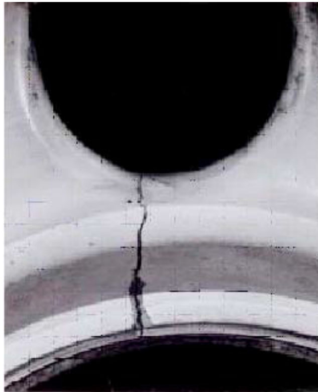
Figure 2-15. Stress Corrosion Cracking
