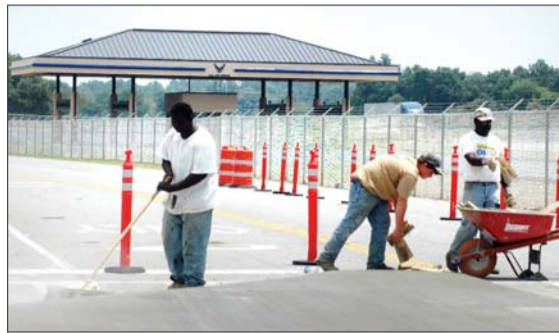
Workers from C.T. Bone Company work on a traffic island at the Martin Luther King Jr. Boulevard gate Monday. The gate is set to reopen Monday.
