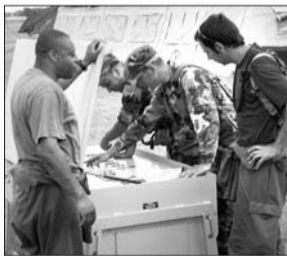
U.S. Air Force photo by GEORGE JOZENS Power production specialists from both the U.S. and U.K. Air Forces work on electrical distribution from their generators.
